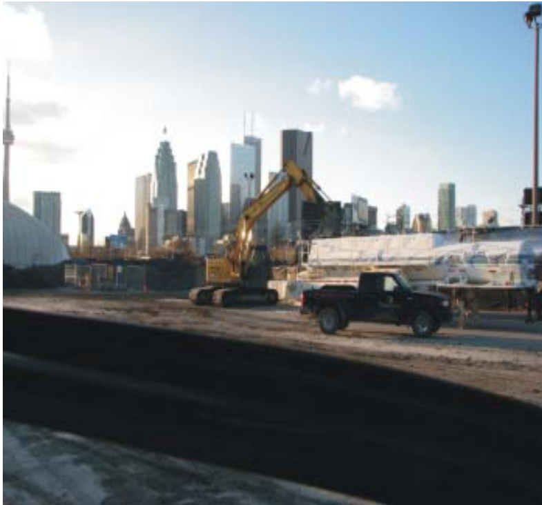
View of site with soils being loaded. The close proximity of Lake Ontario (foreground) necessitated that a dewatering program be implemented during the soils excavation.
