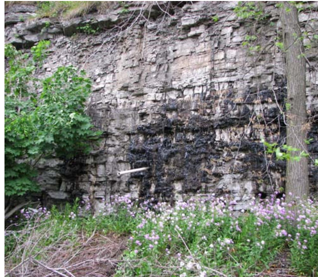
Rock face with Bunker C leached through rock face.
