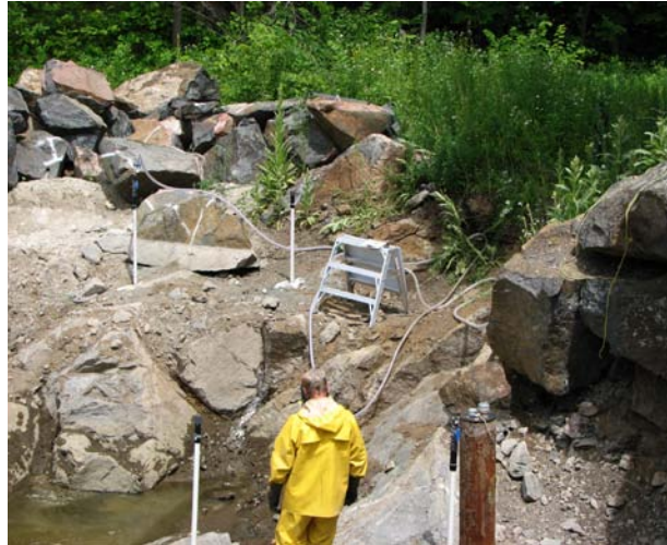
Injection wells installed in bedrock in the footprint of the former residence
