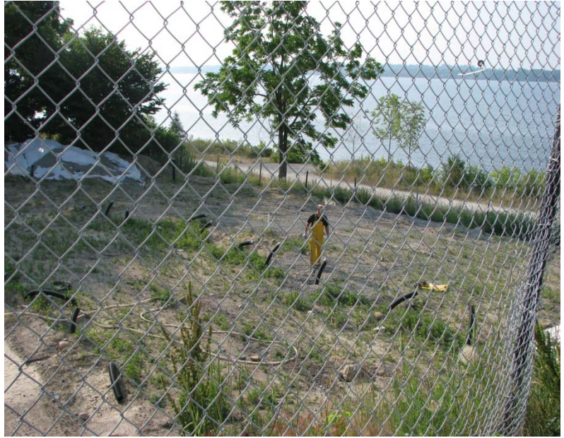
In-situ remediation with Big O injection wells installed in preparation for OxyTek-L™ injection
