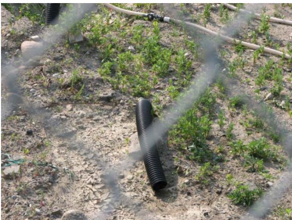
Big O tile injection well
