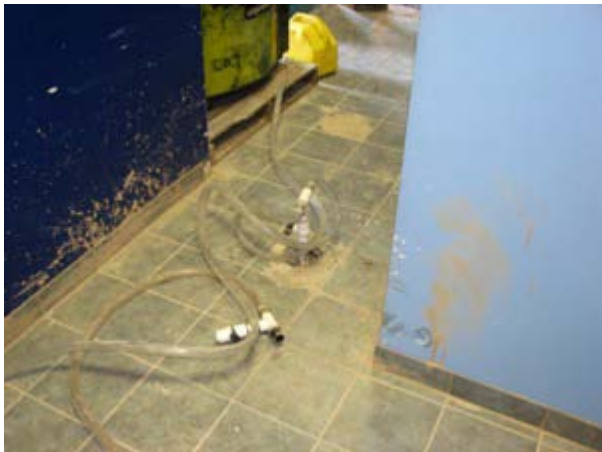
OxyTek-L™ was injected into wells in the office area of the building
